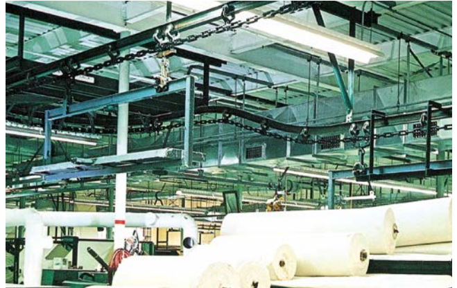
Trolley conveyor system
